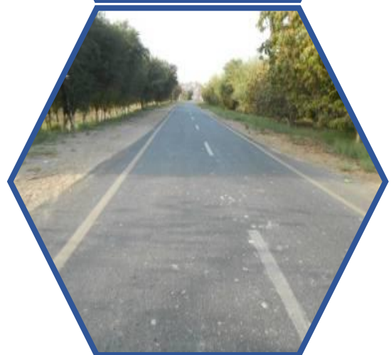
W/R of road from Saddiq Memon to Hafiz Sandhano road to Tando Allahyar
