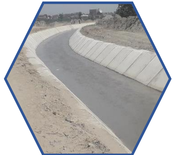
C.C. Lining of Wagherji Distry
