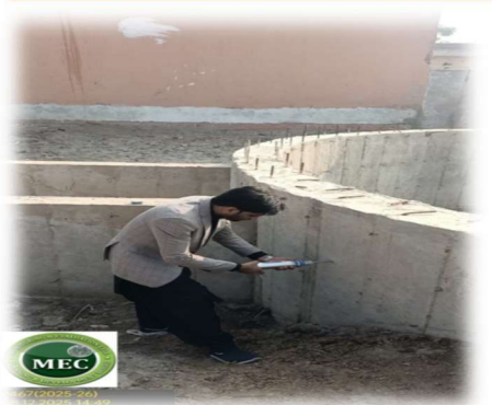
Conducted rebound hammer tests on the constructed collection tank using a Schmidt Hammer
